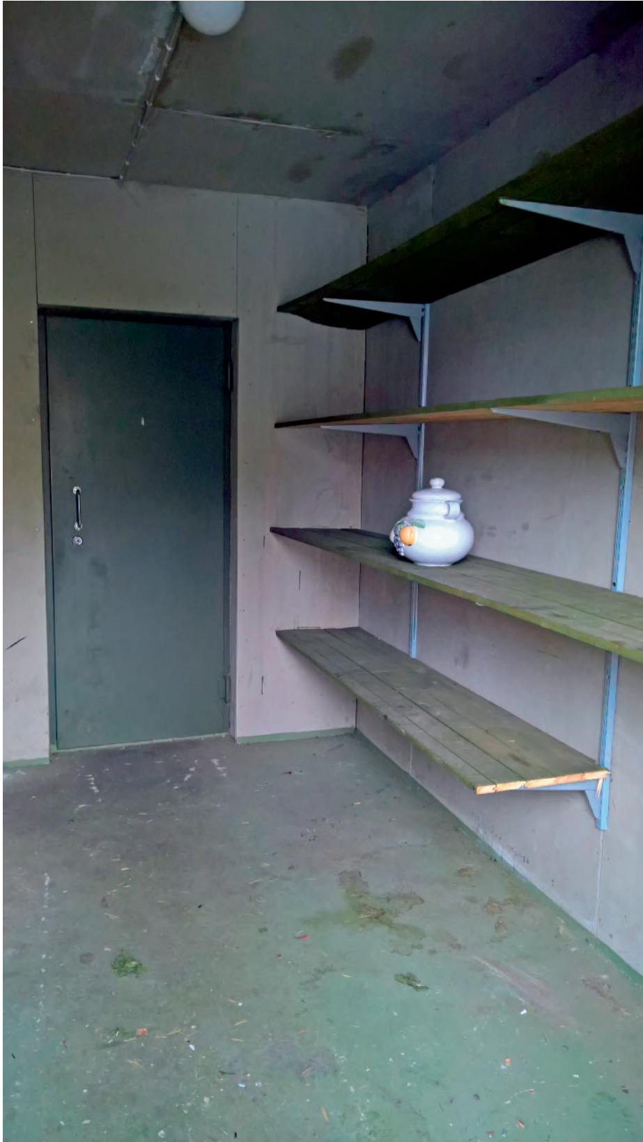
Figure 11.9. A lone burial urn in the house storage waiting for transportation to the Mikonkangas pet cemetery. Note the stains on the ceiling that record a substantially long history of roof leaks.
