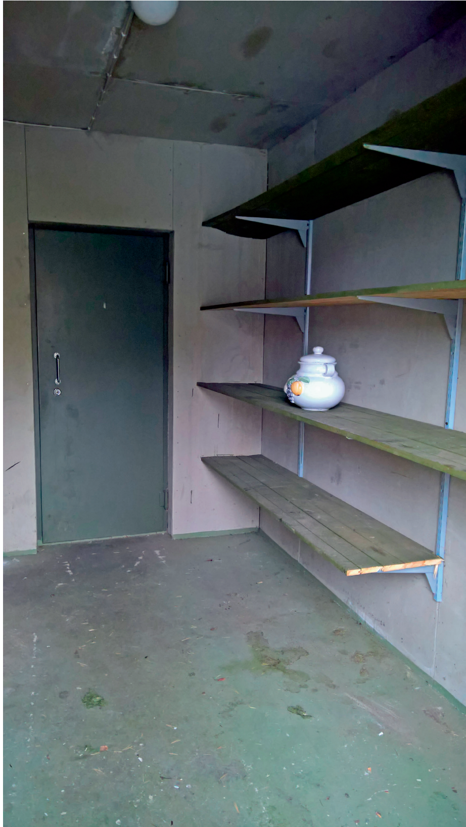
Figure 11.9. A lone burial urn in the house storage waiting for transportation to the Mikonkangas pet cemetery. Note the stains on the ceiling that record a substantially long history of roof leaks.
