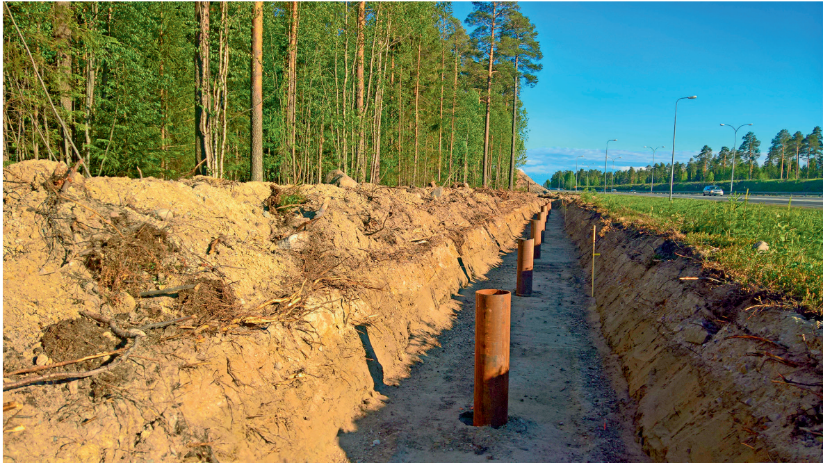
Figure 11.16. The foundation trench needed for the installation of a sound barrier caused a deep temporary scar on the western side of the Hiironen pet cemetery.
